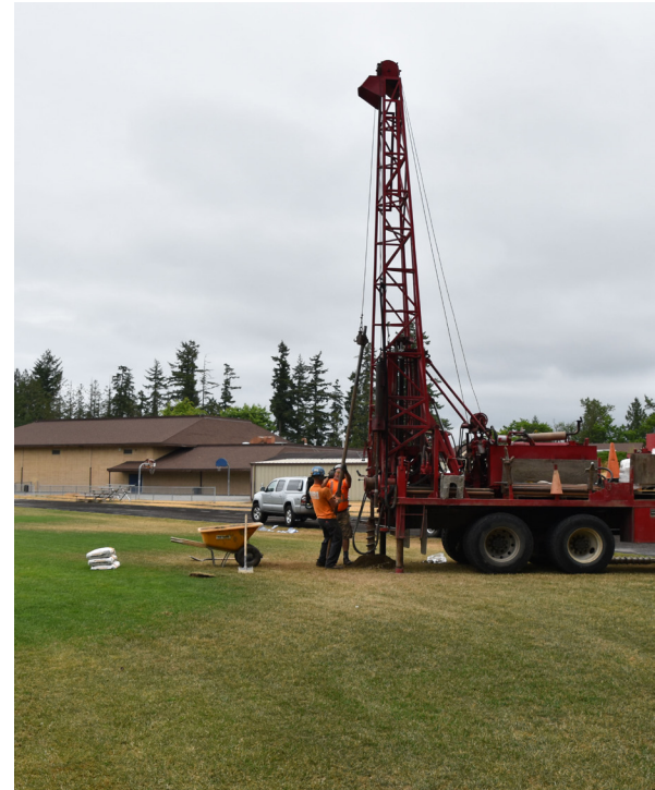
Over the summer, drilling took place near Post Middle School to ensure the soil could safely accommodate the building of a new middle school on the site.
